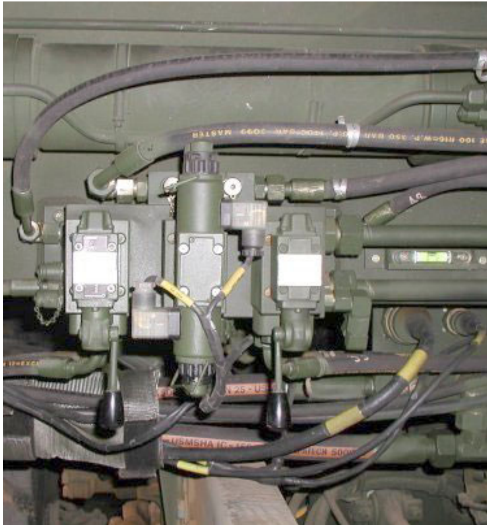
Figure 3. 22 A-frame Stabilizer Controls
